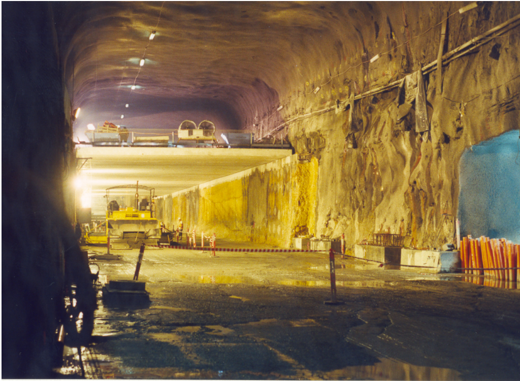
Photo 2 Concrete planks for Northbound Lanes supported on narrow ledge – approaching fault zone wherein the planks had to be supported on a column-beam structure
